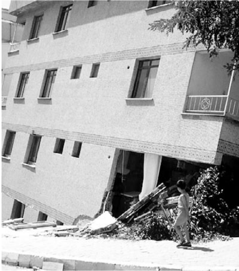
Earthquakes can damage or even destroy buildings.
