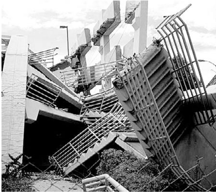
An earthquake destroyed this building.
